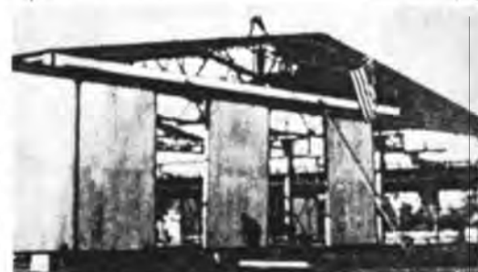
This hangar was under construction in the Fall of 1932 at Weeks Field Fairbanks when picture was taken.
